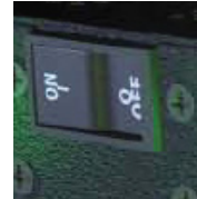
Example: Breaker On
