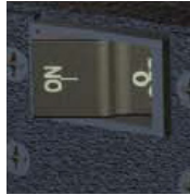
Example: Breaker Off
